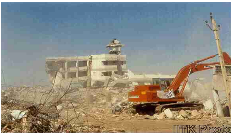
Virtually nothing can be recovered from most RCC frame buildings that collapse. Clearing of debris from numerous multistorey RCC frame buildings is an even bigger challenge.
