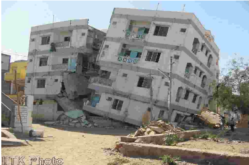
Aftermath of an earthquake: even RCC frame buildings can break apart!
